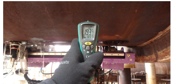
Elevated surface temperature
